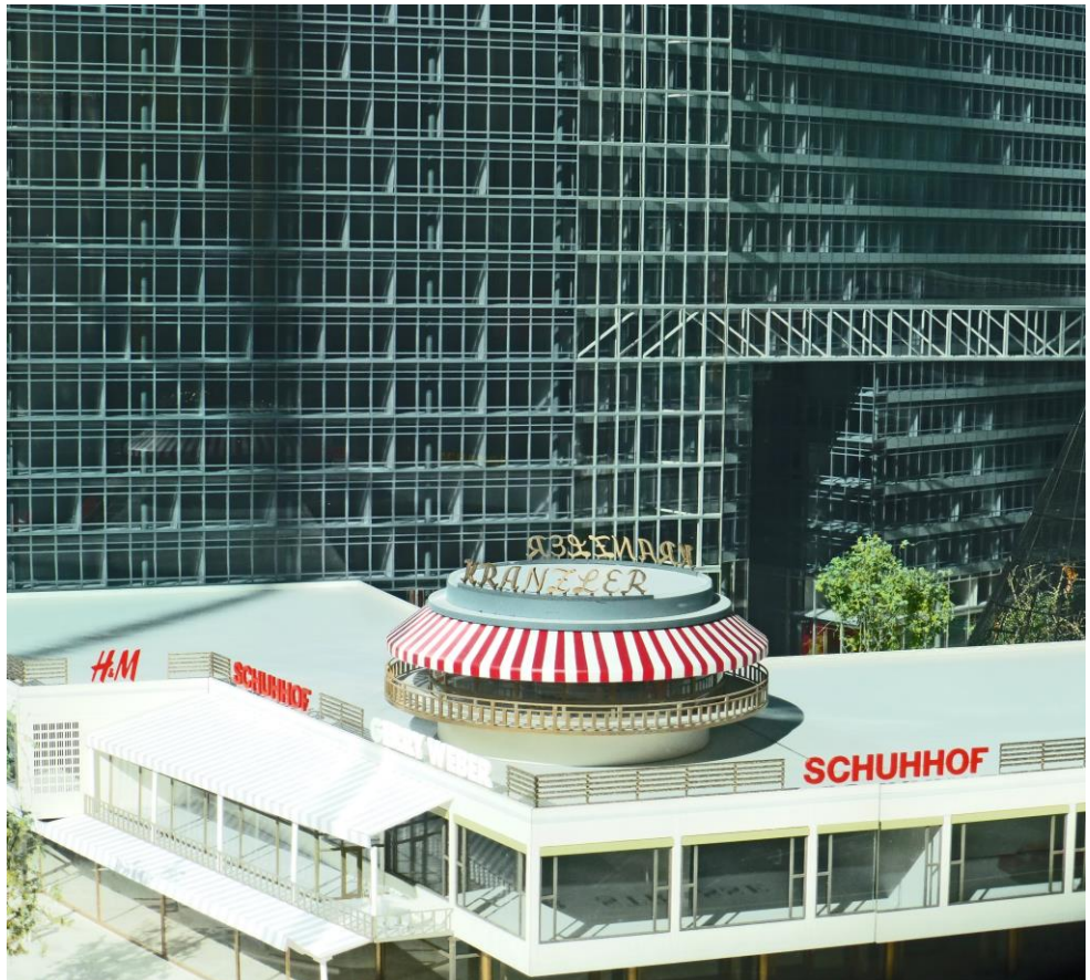
The Neues Kranzler Eck building in Berlin under construction, showing the pultruded frames installed prior to glazing.
