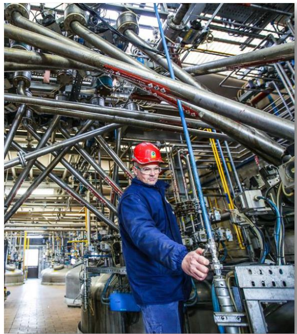
At AOC's Filago plant, audits, monitoring programmes and investigations by a dedicated project team identified various ways to reduce energy consumption and associated CO 2 emissions. (Image @ AOC.)
