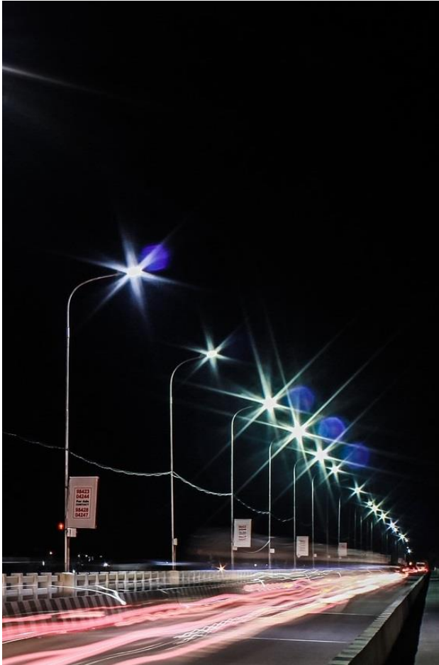
The humble street light is evolving into a platform for delivering smart city services.
