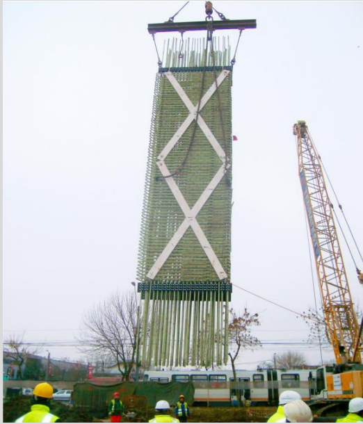
Installation of a soft-eye structure during the construction of a metro line in Bucharest.
